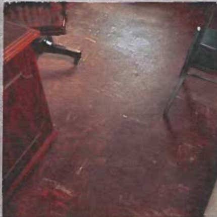
Nine-inch floor tiles in rear addition, likely containing asbestos.
