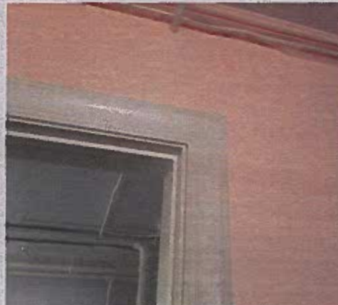
Present-day condition of painted wood trim.
