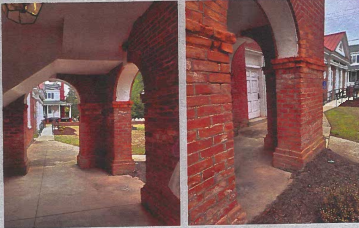
Sussex County Courthouse today showing advancing masonry damage at the piers of the East portico.
