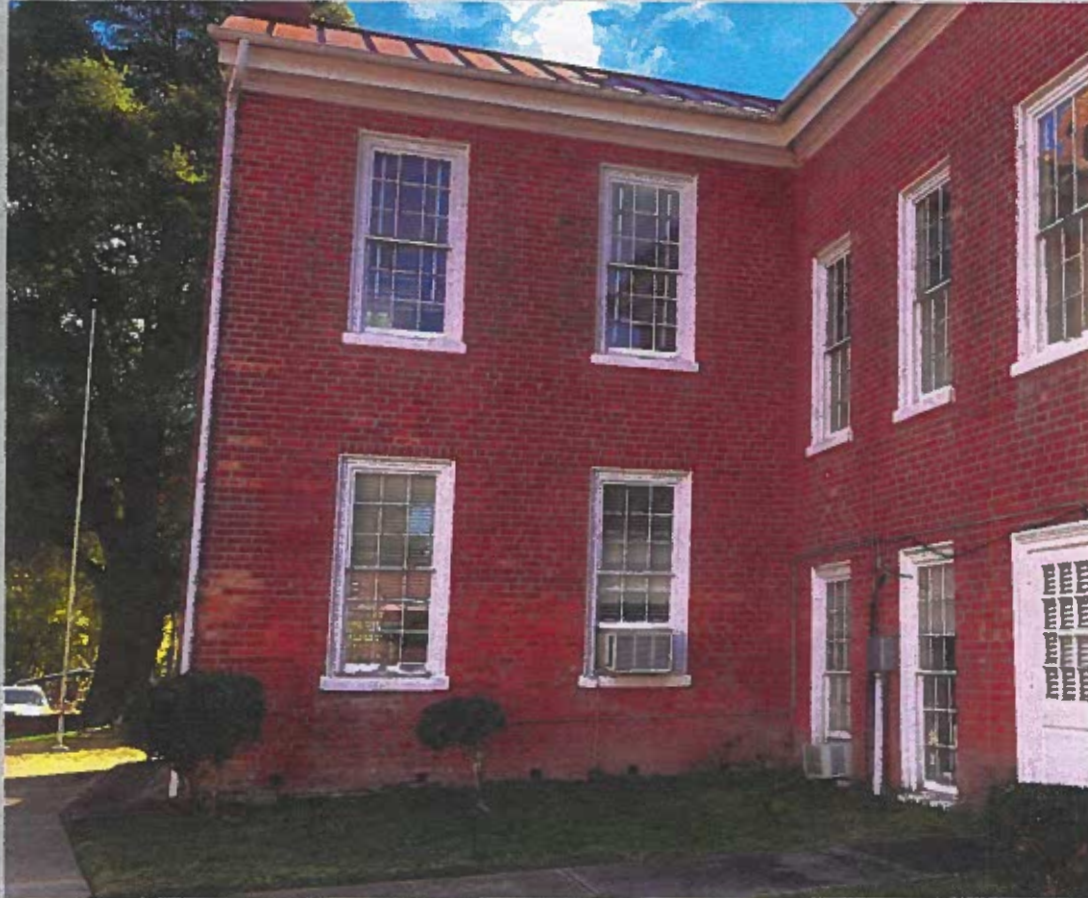
Northwest corner of original courthouse highlights some of the mysterious discrepancies around the placement of its windows.
