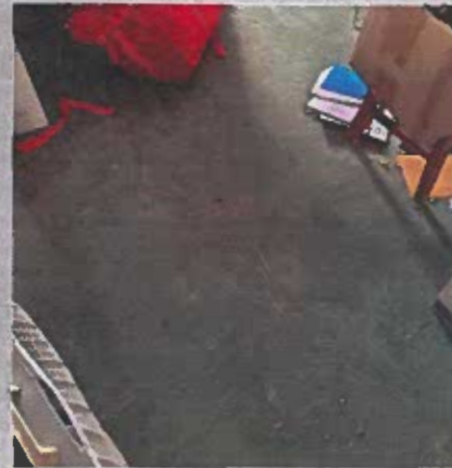
Nine-inch floor tiles in rear addition, likely containing asbestos.
