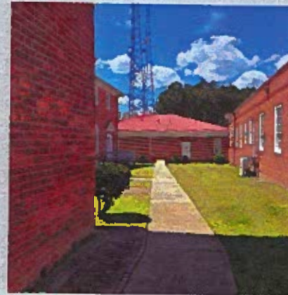
Brick conditions on north wall parallel to walkway.
