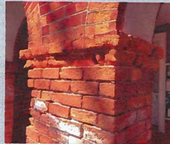
Sussex County Courthouse today showing advancing masonry damage at the portico.
