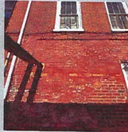
Brick condition within open-air mechanical yard.
