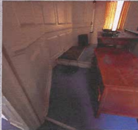
Curved wall in courtroom covered in 1954 paneling concealing the original central window.
