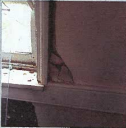
Plaster deterioration condition near window.
