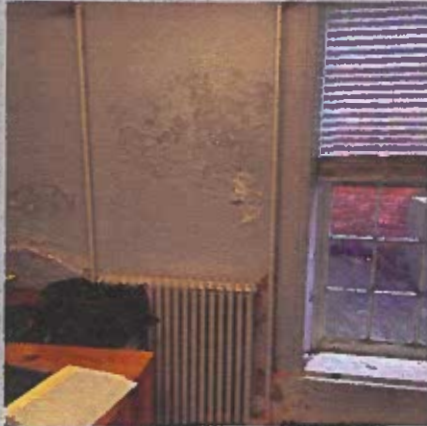
Paint delaminating near window on ground floor.
