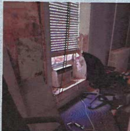
Plaster deterioration and paint delaminating in original courtroom.
