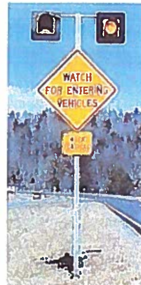
Figure 7: Actuated Flashing Beacon
