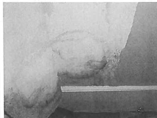
Photograph 4: View of significant mold growth behind wallpaper on the 1 st floor
