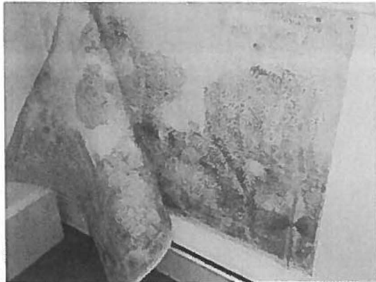
Photograph 1: View of significant mold growth behind the wallpaper on the 1 st floor
