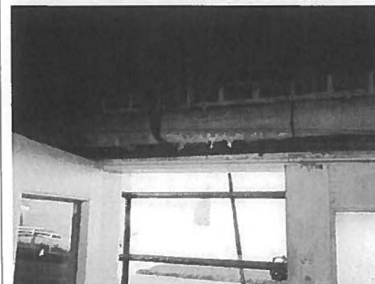
Photograph 6: View of ACM (pipe insulation) in the basement
