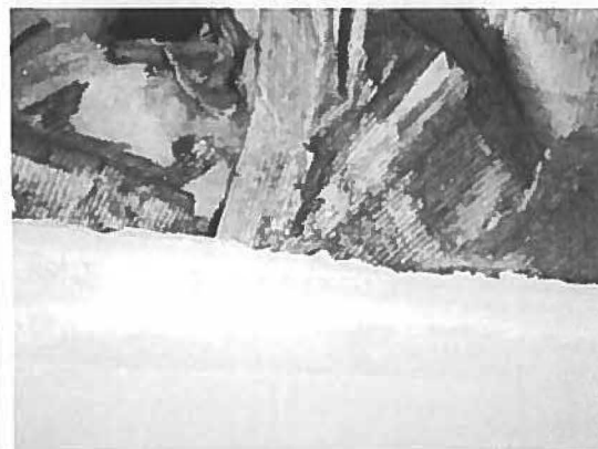
Photograph 3: View of mold growth on insulation in the ceiling of the 1 st floor
